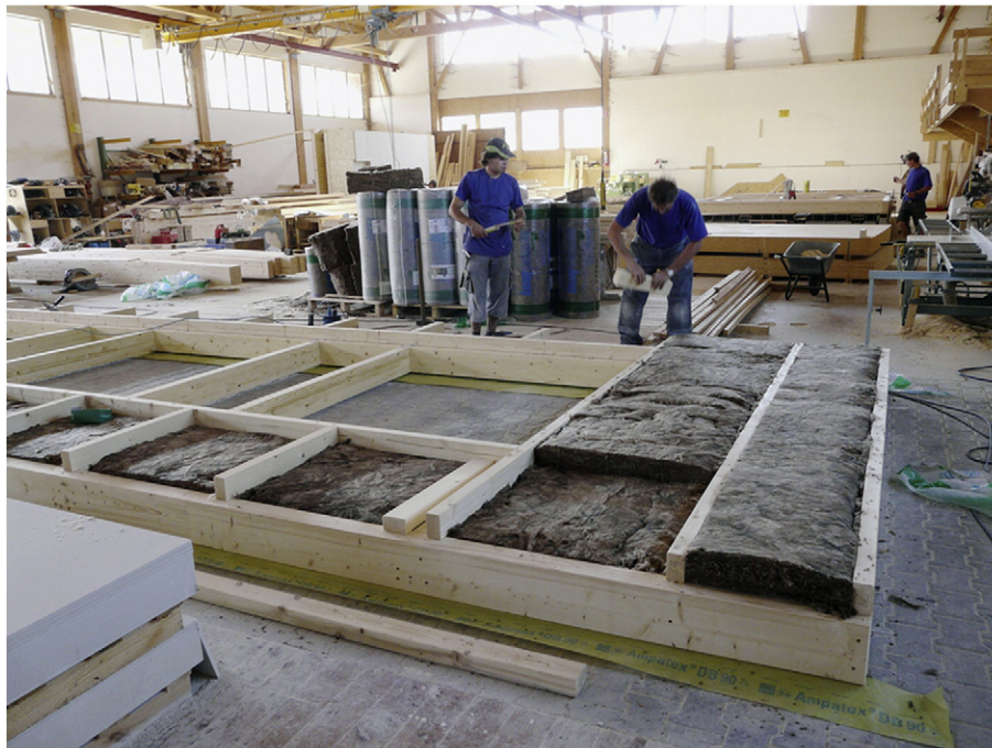
Fig. 2. Prefabrication of the elements in the factory for the college of Buchloe, Germany.
