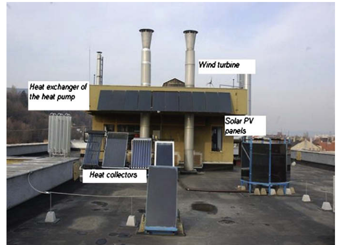
Fig. 1. Budapest Tech renewable system.
