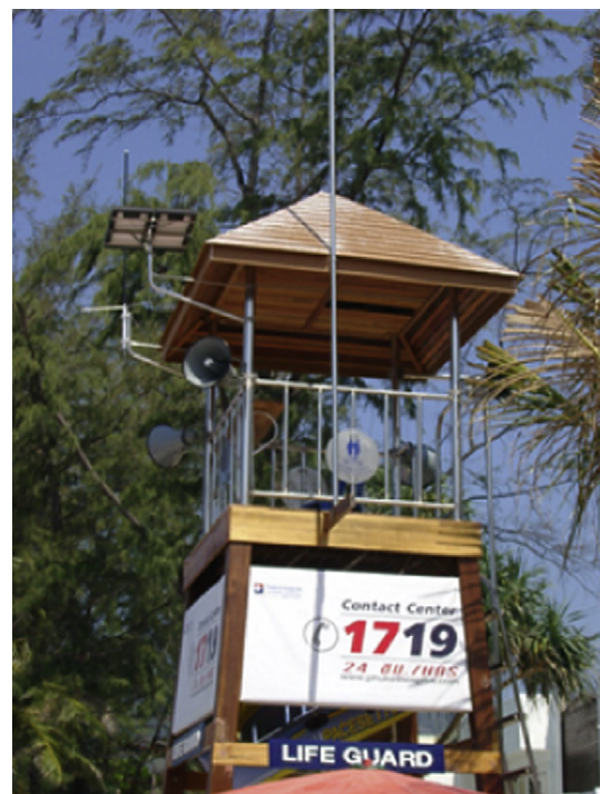
Fig. 1. Part of the tsunami warning system at a tsunami-hit beach in Thailand.
