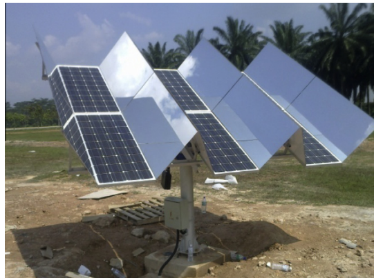
Fig. 1c. Installed CPV system with mirror concentrating elements.
