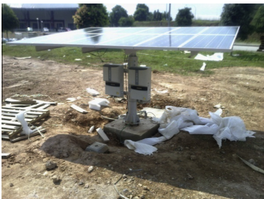
Fig. 1a. Installed fixed flat PV system.
