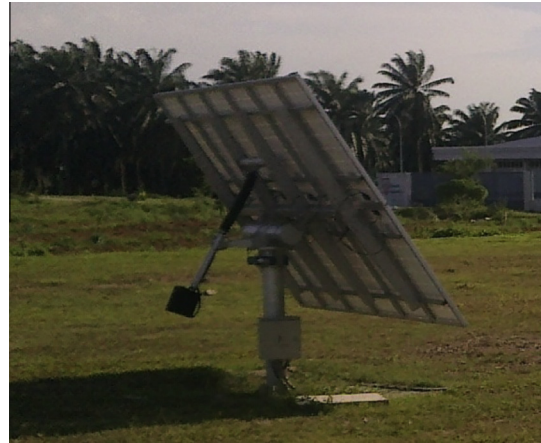
Fig. 1b. Installed tracking flat PV system with 2-axis movement.
