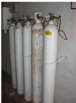
(a) Gas tanks
