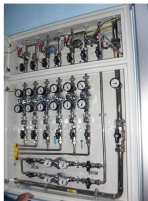
(b) Gas control panel
