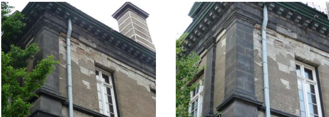
Fig. 2 Deterioration of stone wall surface (left: June 2009, right: October 2011)
