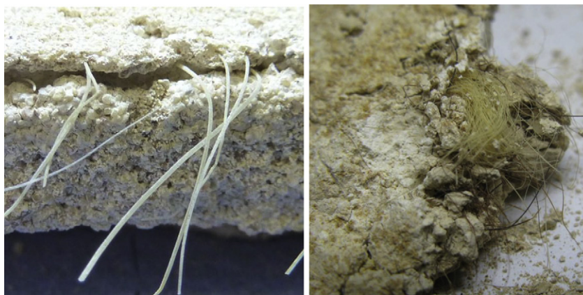
Fig. 1. Hair protruding from a modern failed plaster (left), and from 200-year-old chalk lime mortar (right). The hair from the modern samples was shown to be aligned, stiff and brittle. The sample being taken from new work in a private building in Somerset, England, in which a non-hydraulic lime putty plaster was reinforced with a hair imported from China, with failure of the plaster occurring due to the apparent partial digestion of the hair across the rivets resulting in detachment of the plaster from the walls; the historic hair sample was much softer and more randomly orientated, and was obtained from plaster removed from an early 19th century building on the South Coast of England.
