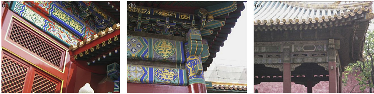
Fig. 1. Three photos showing ‘colour decay’ on historical buildings in the Forbidden City, Beijing: (a) recent repainting during a major renovation of the Forbidden City before the 2008 Beijing Olympics; (b) colours starting to decay; (c) significant colour degrading.
