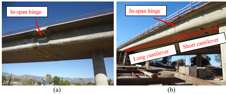
Fig. 1. (a) In-span hinge of CIP/PS box girder bridges (N170-N5 Connector, Los Angeles); (b) hinge span (Del Paso Park Overhead, Sacramento).
