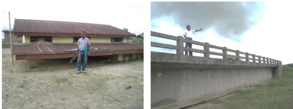
Fig. 1. An abandoned building and an R.C.C bridge due to sand casting. (deposition of the coarse fraction of the load over the flood plains).
