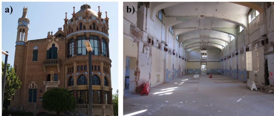
Fig. 1. (a) Photograph of Sant Manuel pavilion nowadays and (b) general view of ground floor at the beginning of restoration.
