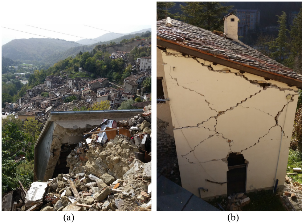
Fig. 1. (a) Collapse of historical building-Pescara del Tronto, Italy; (b) shear damages of a building in Visso, Italy, 2016.
