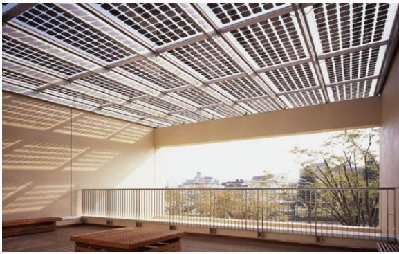
Fig. 1. An example of BIPV in which photovoltaic arrays are combined with the roof.
