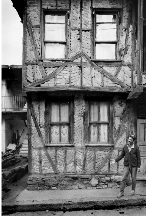
Fig. 1. This long abandoned and unmaintained 2.5 story humuş house in Gölcük survived the 1999 earthquake with little additional damage, despite the widespread collapse of the surrounding RC structures.
