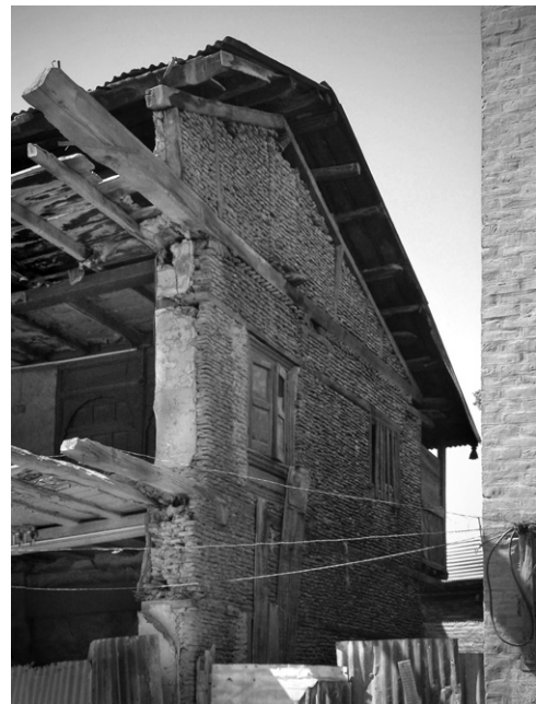
Fig. 3. Partially demolished taq construction (Srinagar, Kashmir, 2006) showing timber lacing laid into the wall. Timber bands at floor level and at the window lintel levels.
