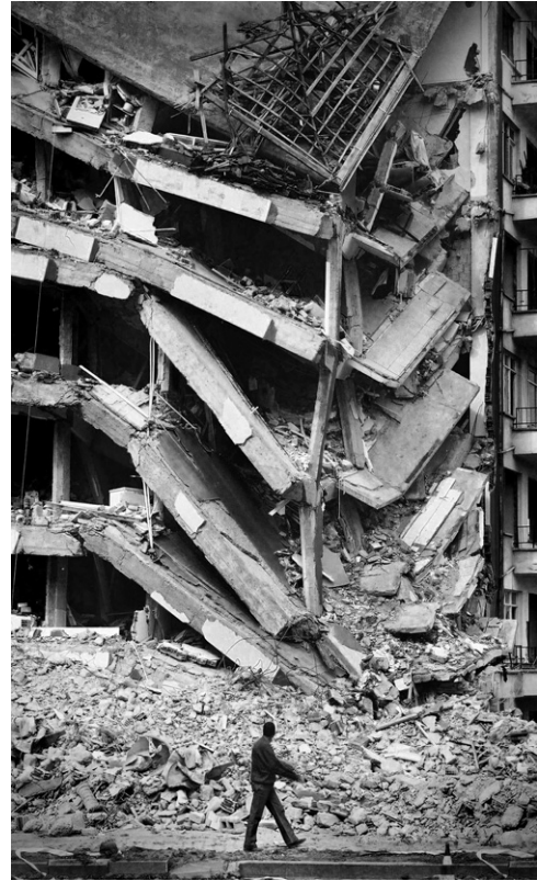
Fig. 2. Partially collapsed RC frame with infill masonry apartment block, Gölcük, Turkey, 1999.
