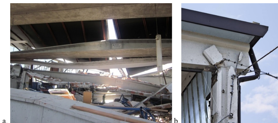
Fig. 1 (a) Damage caused by the collapse of the roof in a RC precast industrial building in Emilia, 2012 (b) failure of the fork at the top of the column due of the out-of-plane stress of the beam.
